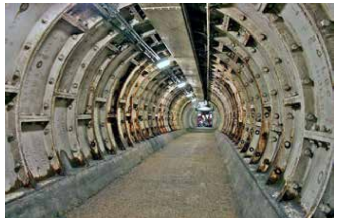
The repaired section of tunnel looking north towards the lift. Photo Mike Peel
